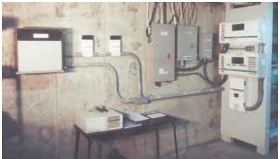
L–R: Dump load, two Trace C-40 shunt regulators, utility grid breaker, AC subpanel, grid/RE transfer switch, Trace 4048 and 5548 inverters with DC 250.
