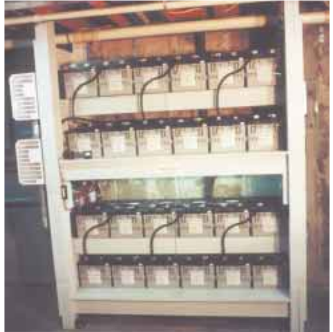
Twenty-four Concorde SunXtender sealed absorbed glass mat batteries provide 1,800 amp-hours at 48 VDC.
