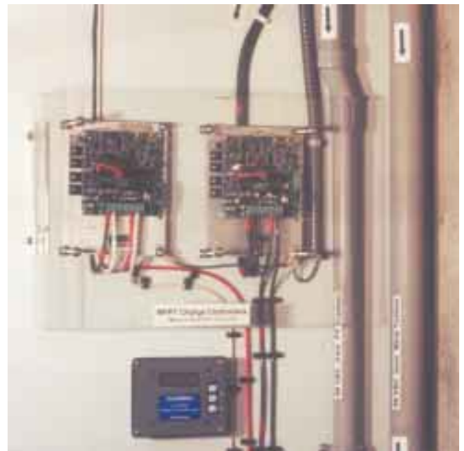
Two MPPT charge controllers prevent overcharging by the two roof-mounted PV arrays.
